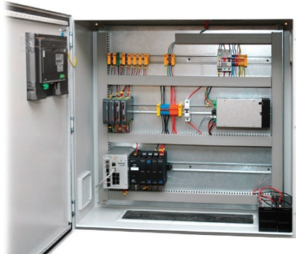
Pict.1 Example of a fire panel
